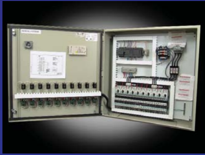
A typical motor control panel with the temperature controller for the Tower Tech 10-fan Modular Cooling Tower
